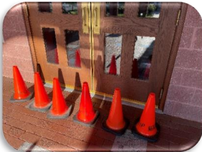
Fixing Front Doors Hanns and volunteers are fixing the church doors. This time it will be better and attractive.
