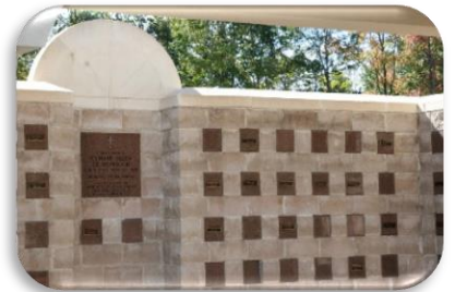
Washing of the Columbarium We are in process of power washing Columbarium #1.
