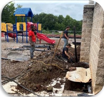
Foundation of Columbarium #1 Installation of ram jacks under the Columbarium to fortify its structure.
